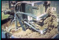
Electrical utility housing
